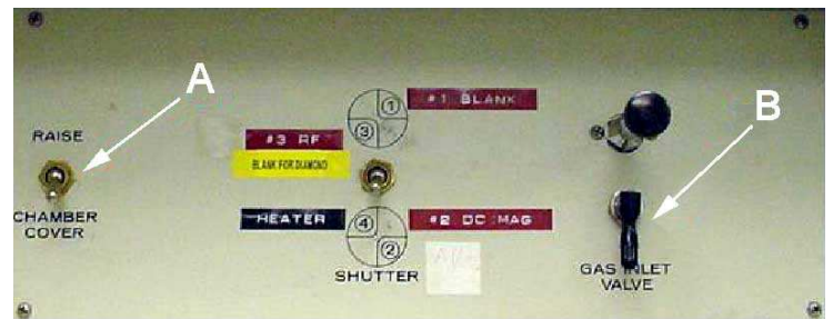
Fig. 2. Chamber and Gas Control Panel
